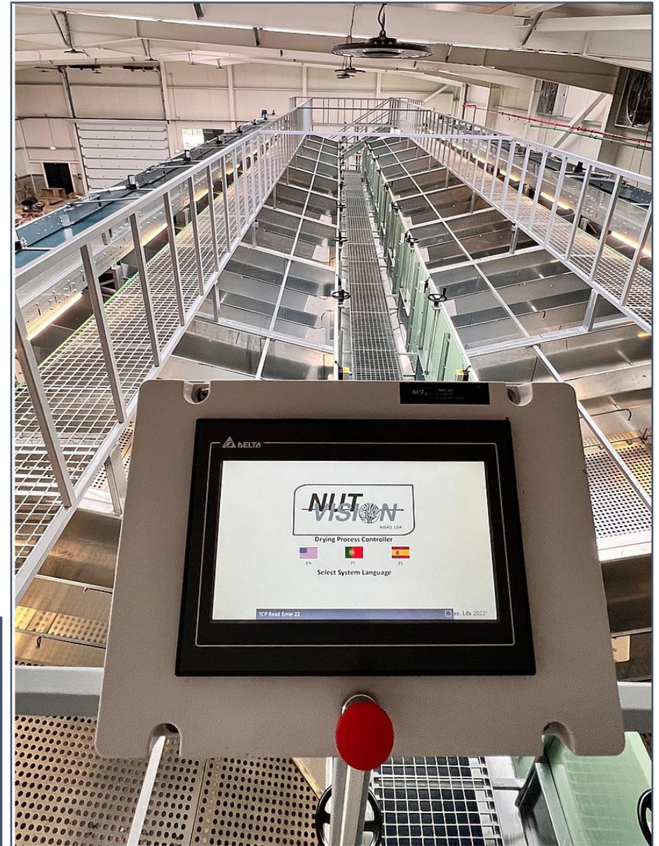
DPC - Drying Process Controller on second level platform
