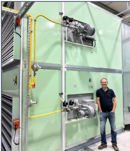
Lower Primary Heater (burner) and the upper Secondary Heater (burner)
